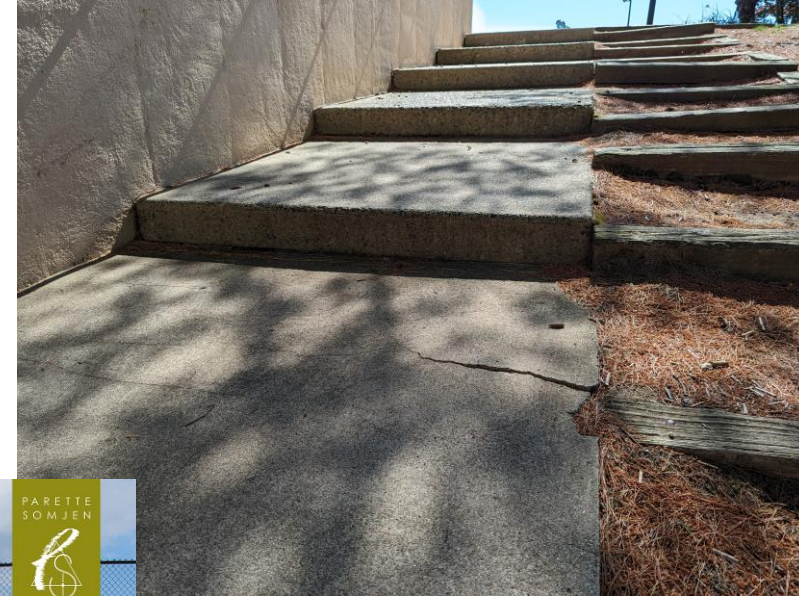
Concrete and railroad tie steps along pedestrian wall up to stadium field
