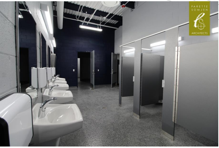
Example of bathroom upgrade, e.g. new touchless fixtures, stalls, floor
